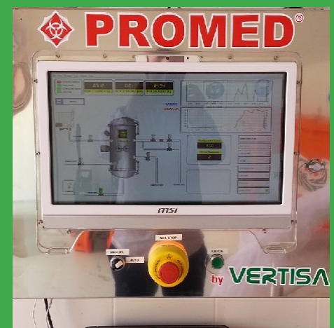
PROMED CONTROL PANEL
